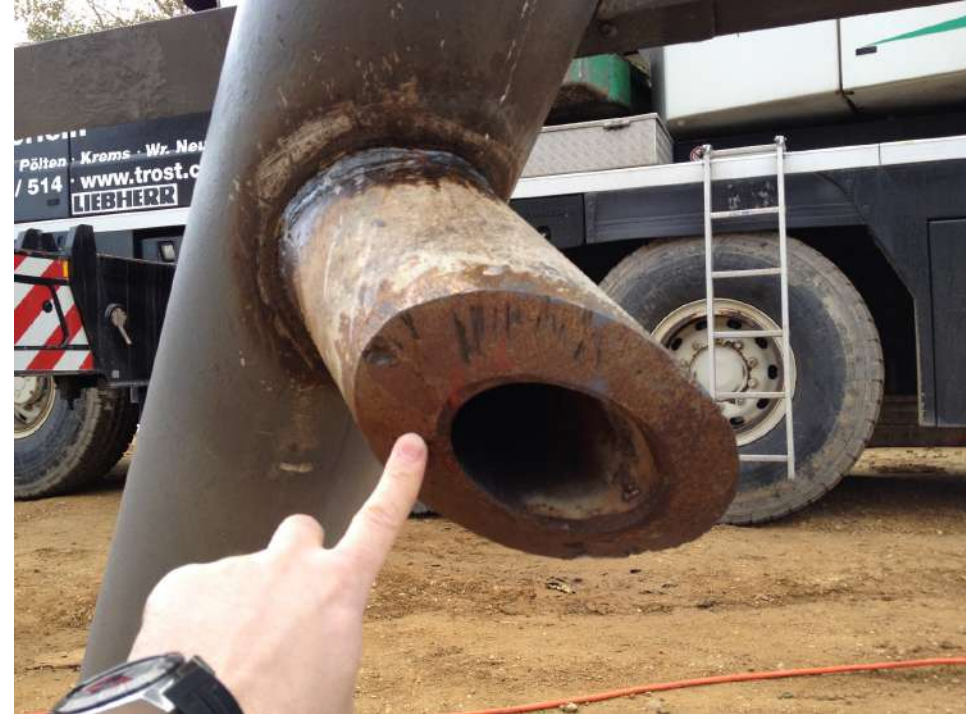
Attachement steel pipe
